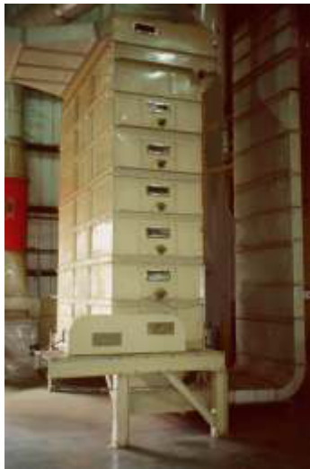
Gin Installation with Rectangular Piping
